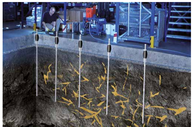
Spreading injection agent, working in open terrain and under existing floor slabs
