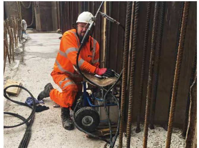
Sealing injection with ram injection lances between bored pile and sheet pile wall
